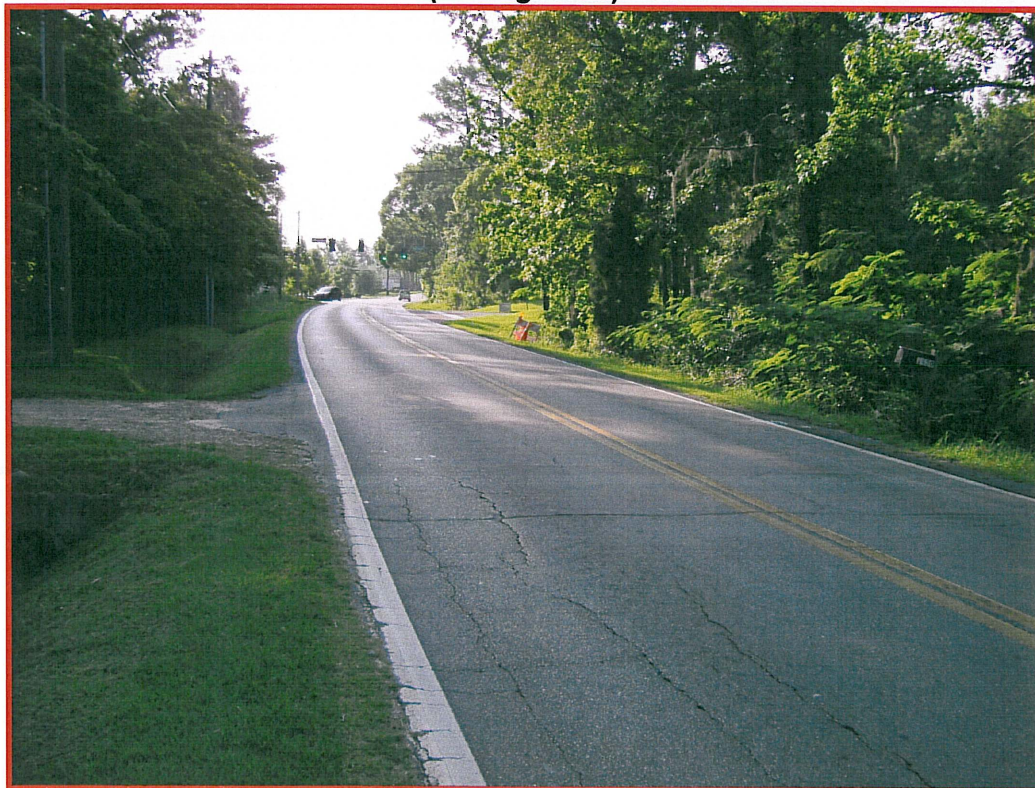
Figure 8: Photograph of Severe Longitudinal Cracking on Bannerman Road (Facing East)
