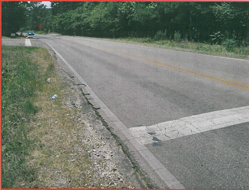
Figure 7: Photograph of Severe Spalling Along Pavement Edges - Bannerman Rd (Facing West)
