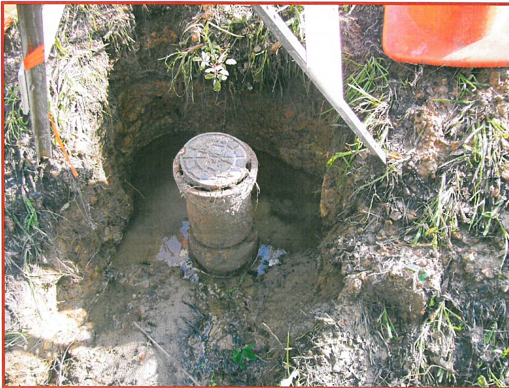
Figure 6: Photograph of Leaking Water Main - Near Soil Boring BH-4
